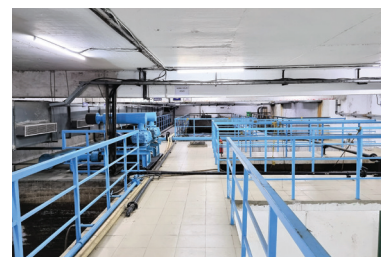
Interior view of an STP at GIPC.
